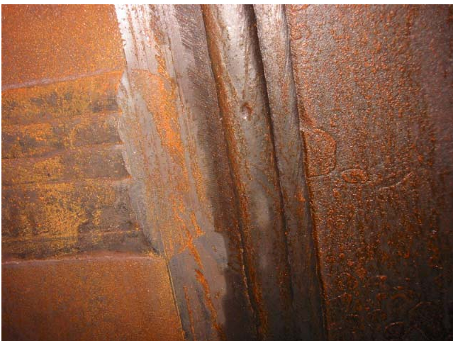
All SAW welds were acceptable in size and profile.
