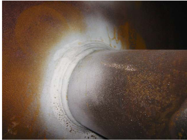
Downcomer nozzles were MPI tested.
