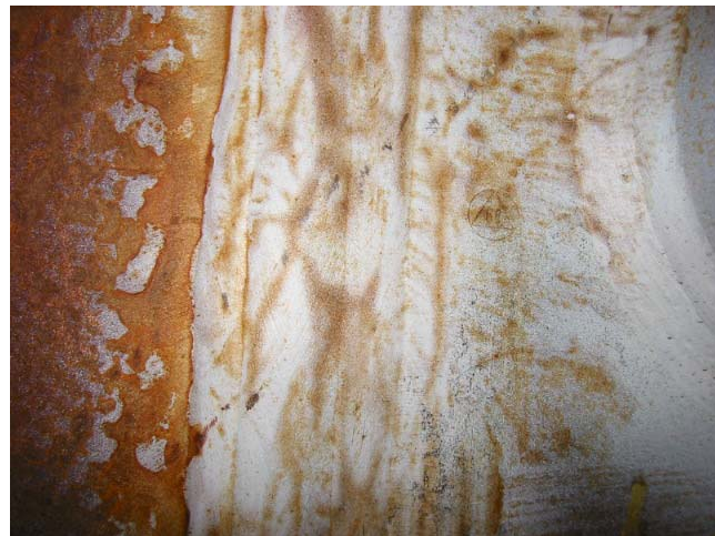
Some minor undercut required grinding.
